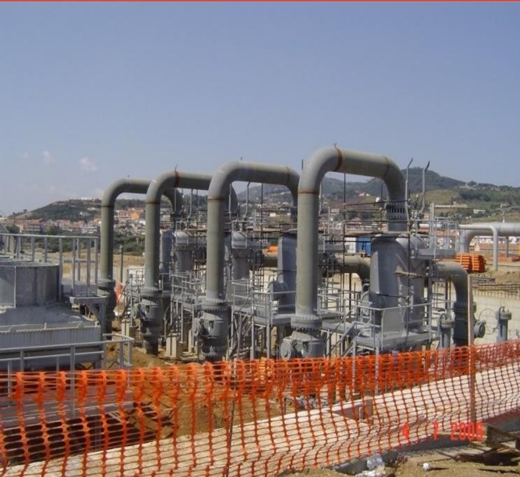
Project: Gas compression station 4 x 25 MW Upgraded turbo compressors, Messina, Italy
